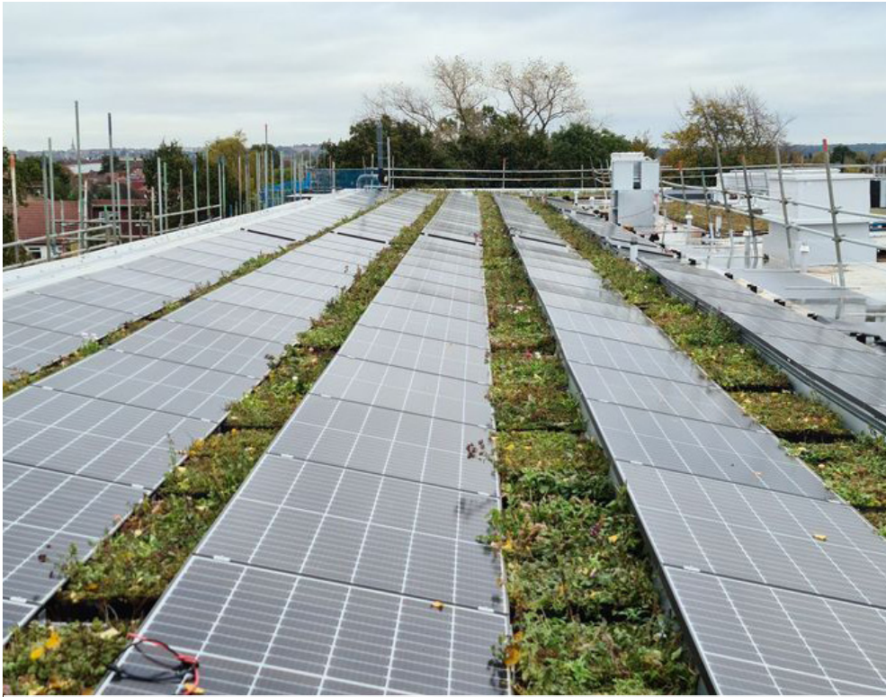
Solar PV panel with green elements, South West London
