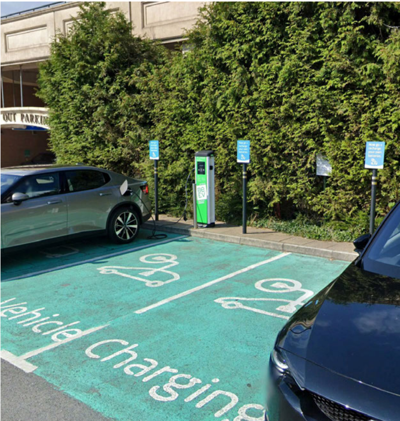
EV charging points, Telford Centre
